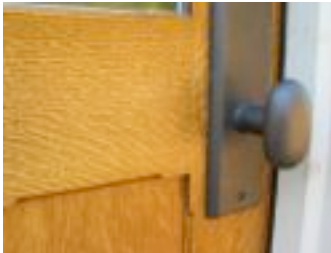
Close up of door hardware on Chris Kovacs' door. Yes, the door is finally hung.
